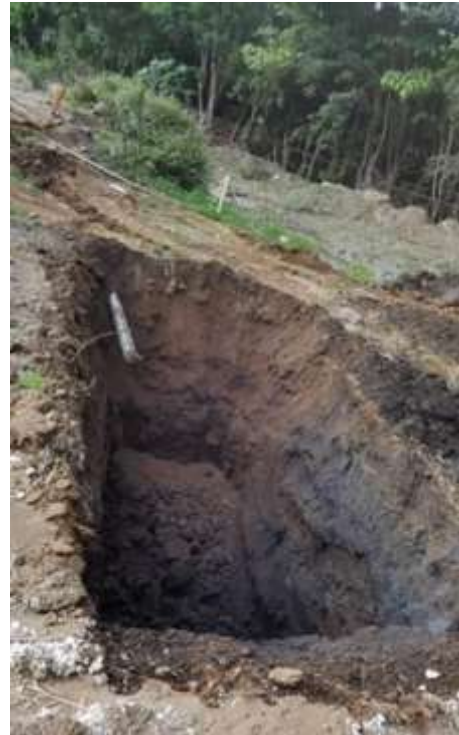
Photo N° 10: T-2 between the trench T-1 and the road. Earth fill, depth excavation 2.5 m. saturated clays
