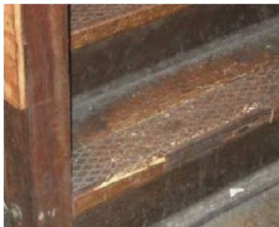
The repair of damaged stairs needs to be a top priority.
