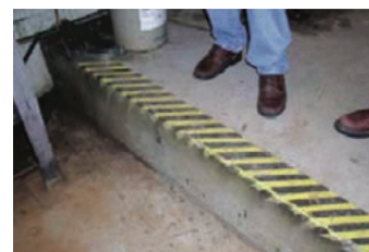
Painting the edge of a single stair to increase visibility can reduce the risk of a stumble and fall.
