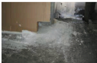
At the door to this walk-in freezer, ice regularly collects on the floor. A thorough assessment of the work area can identify potential problem areas and allow management to eliminate the issue or implement procedures to reduce the risk.
