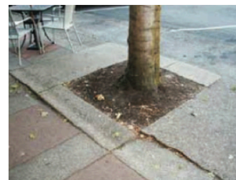
Raised concrete, pavers, and bricks create a trip hazard. Tree roots can raise sidewalks and walkways when a tree is planted too close.
