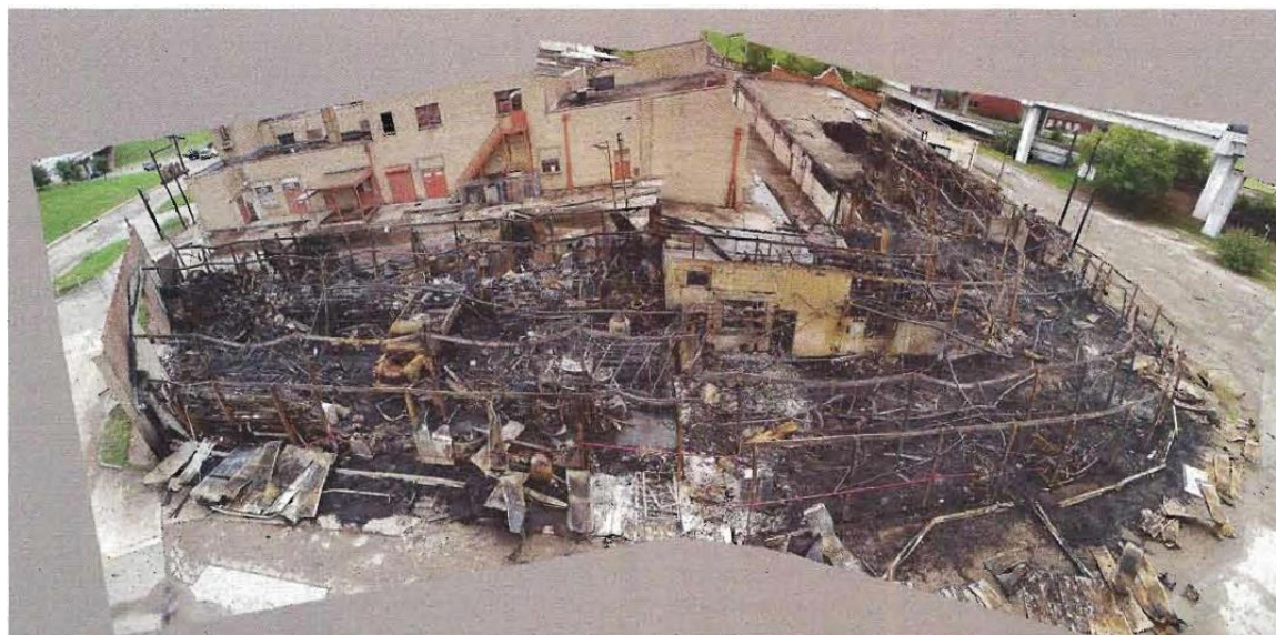
Figure 13-2 Mosaic of warehouse burn scene from aerial truck.
