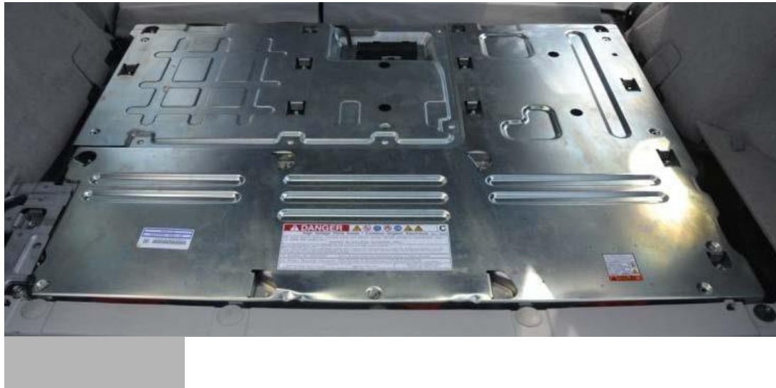
Figure 8 Battery A compartment in cargo area with carpet and molded plastic cover removed
