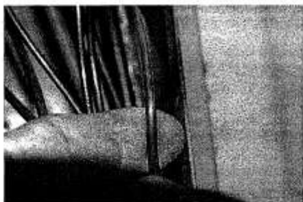
Figure 8-13 Ground fault from damaged (cut) insulation.
